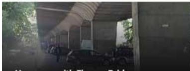
Hammersmith Flyover Bridge Post-Tension Tendon Monitoring provided by MISTRAS
